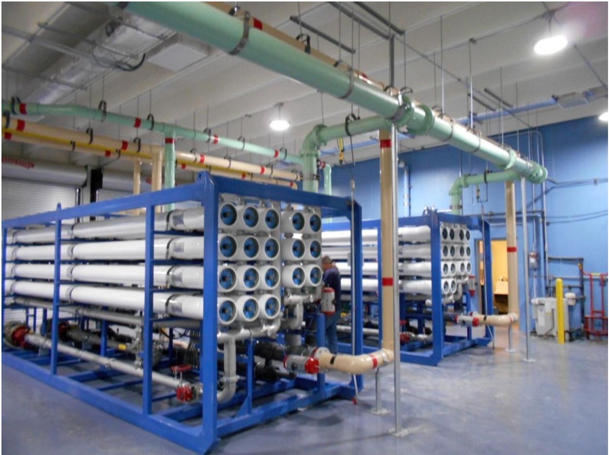
FIGURE 2.2.3.1. REVERSE OSMOSIS FACILITY
