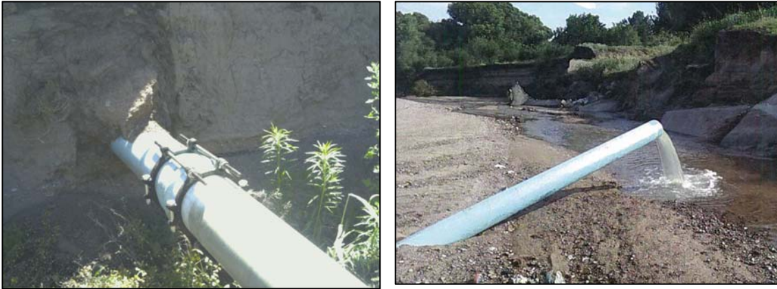
Figure 3 EXPOSED FORCE MAIN AT POTRERO CREEK
