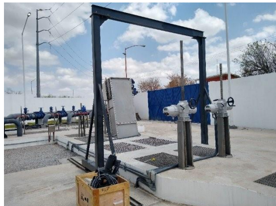
Lift Station No. 278
