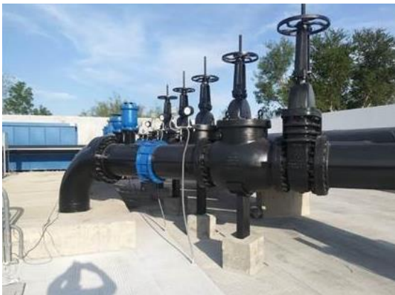
Lift Station No. 1
