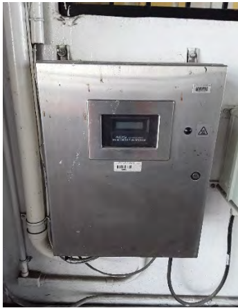
Photograph 45: effluent meter from PB1A
