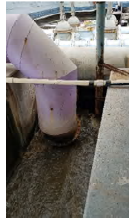
Photograph 22: drop pipe into inlet channel
