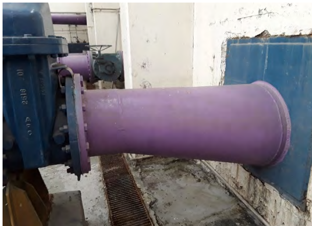
Photograph 29: reducer from inlet channel into pump rain 3
