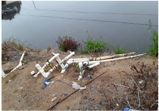
Photograph 16: tie-ins to lagoon system
