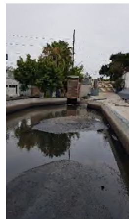
Photograph 12: Sedimentation within inlet channel
