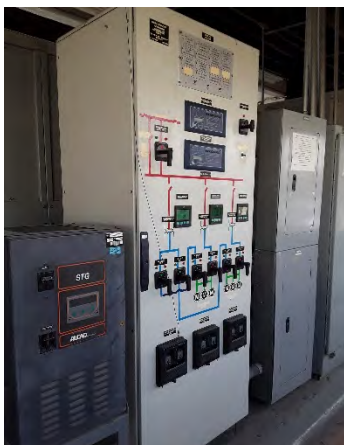
Photograph 41: transformer control panel at PB1A
