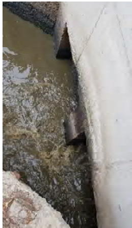
Photograph 21: influent channel into PB1B
