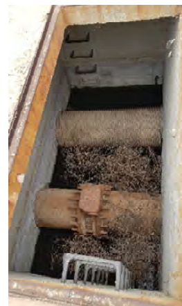
Photograph 24: gate valve at discharge
