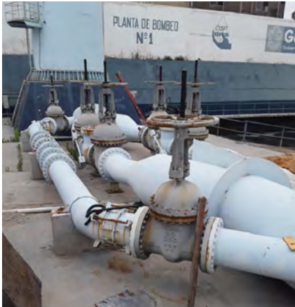
Photograph 13: 20 in gate valve newco
