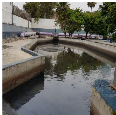
Photograph 6: sedimentation ramp and channel, from International Collector deteriorated conditions at PB1A &B. Trash along the edge of concrete.
