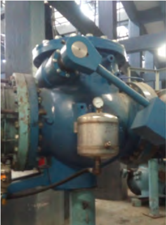
Photograph 40: check valve setup
