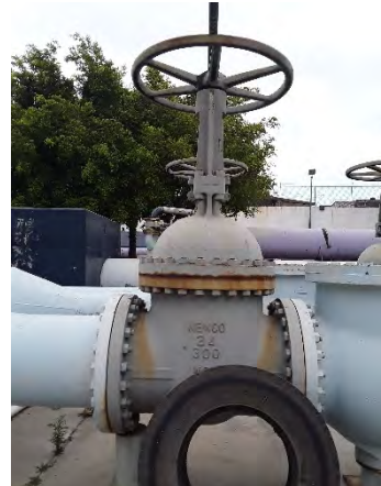
Photograph 14: 24 in gate valves for surge control system
