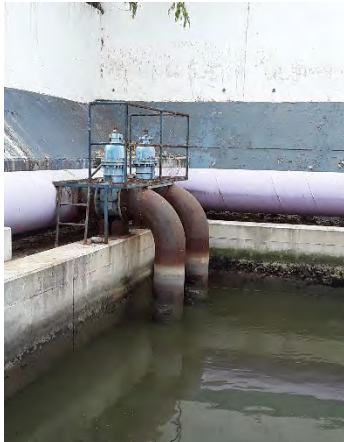
Photograph 1: (2) - 24-inch gate valves from PBCILA, exterior oxidation noticeable
