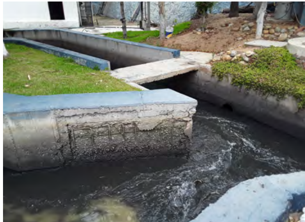
Photograph 3: Sedimentation Channel deteriorated conditions at PB1A &B
