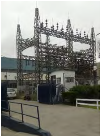
Photograph 42: sub station for both PB1A and PB1B
