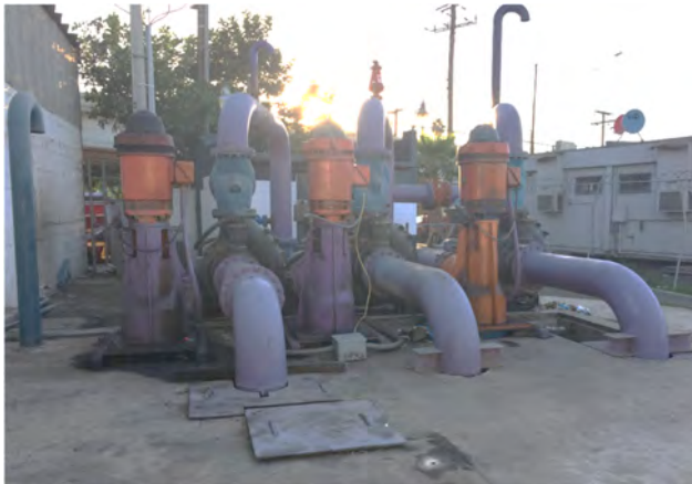
Photograph 1: PBCILA lift station configuration
