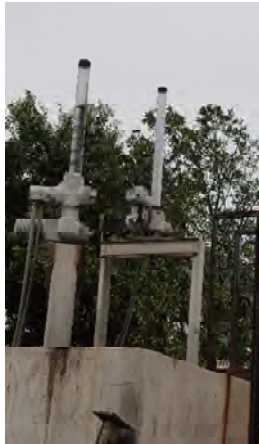
Photograph 13: Gate operating valves
