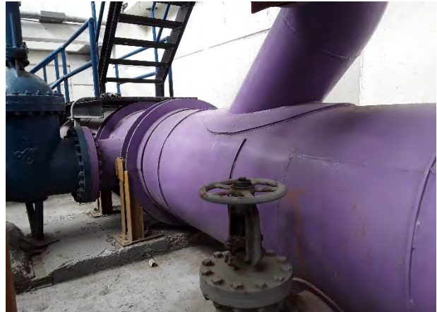
Photograph 20: PB1A effluent manifold
