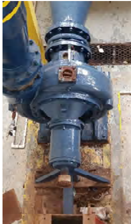
Photograph 7: centrifugal pump at lift station
