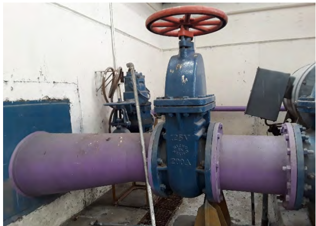
Photograph 30: reducer from inlet channel into pump rain 4
