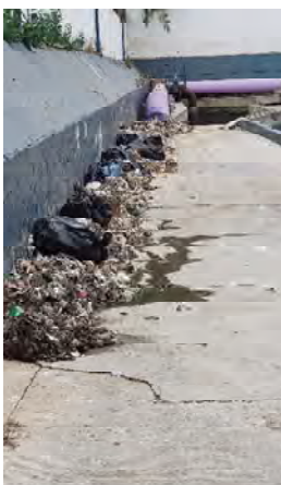
Photograph 53: Trash collected along the side of the lift station
