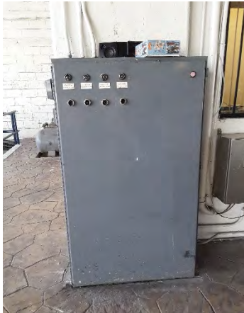
Photograph 43: sump pump control panel
