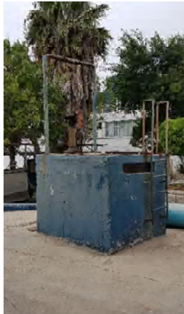
Photograph 7: influent junction box from Sanchez Collector
