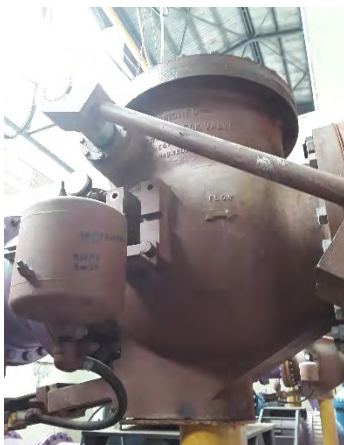
Photograph 11: 20 in mov not operational
