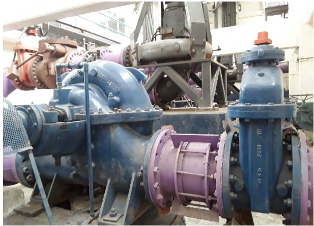
Photograph 28: Pump train not in service at PB1A
