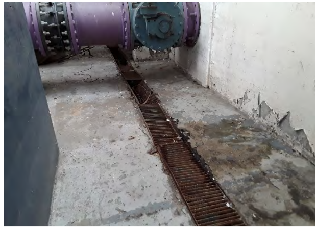
Photograph 22: PB1A effluent manifold and check valve
