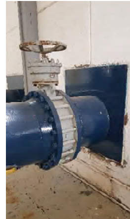
Photograph 14: gate valve at lift station
