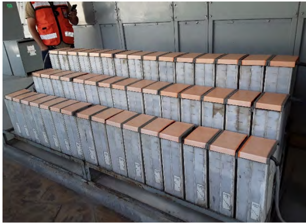
Photograph 39: Batteries at PB1A
