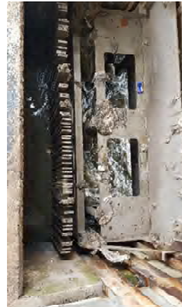
Photograph 50: Trash rack for screens
