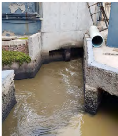
Photograph 5: Inlet Channel, from International Collector deteriorated conditions at PB1A &B
