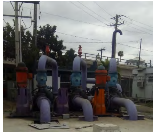
Photograph 4: Pumps 1 and 3 in place, pump 2 decommissioned. Only pump 1 is operational
