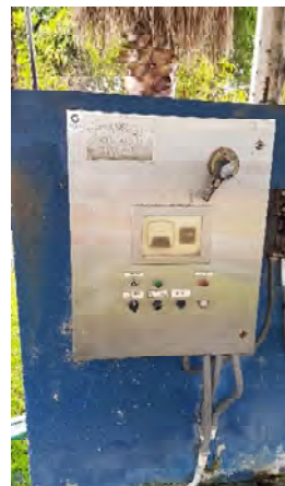
Photograph 4: Control panel for mechanical racks
