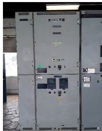
Photograph 36: MCC at PB1A
