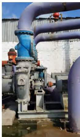
Photograph 5: Pumps 4 to 6, stagnant water from pump 6 air release pipe discharges
