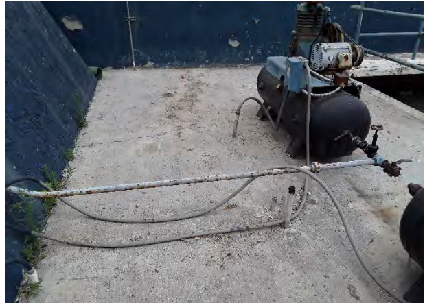
Photograph 2: carbon steel feed line to compressors outside PB1A&B
