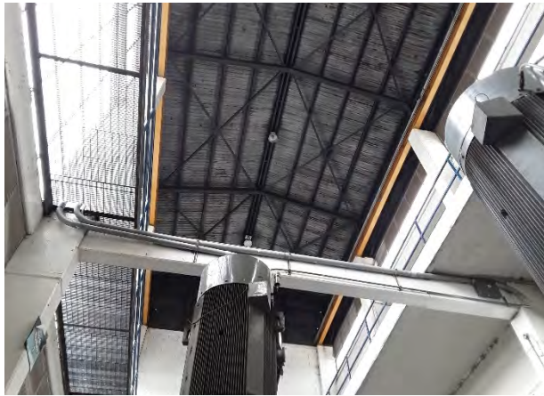
Photograph 27: Train 3, hoist beams and building ceiling
