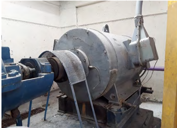
Photograph 31: old centrifugal pump, not in service
