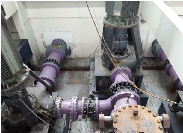
Photograph 33: pump 4 train in service
