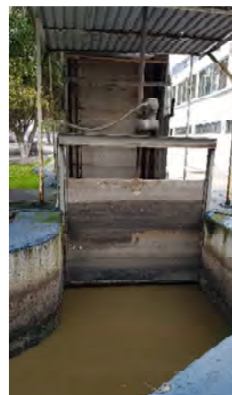
Photograph 6: Mechanical rank channel, metal gate and screens
