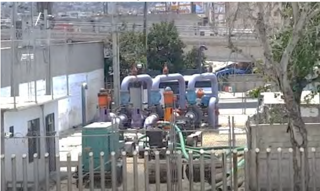
Figure 3-3. View of PBCILA Lift Station
