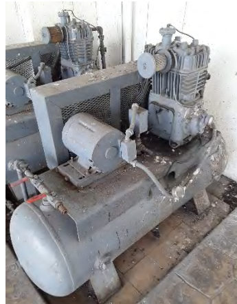
Photograph 44: air compressor at PB1A
