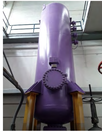
Photograph 34: surge tank at PB1A
