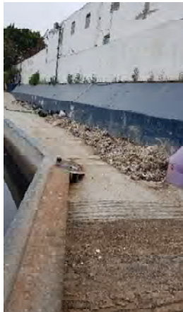
Photograph 9: Trash piles along lift station property
