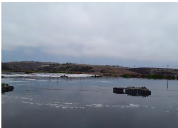
Photograph 17: biological lagoon with non-operational aerators
