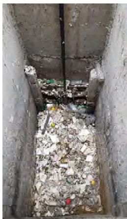
Photograph 17: trash at blocked gate shown
