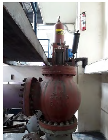
Photograph 12: 24 in gate valve for effluent ww 1 of 2
