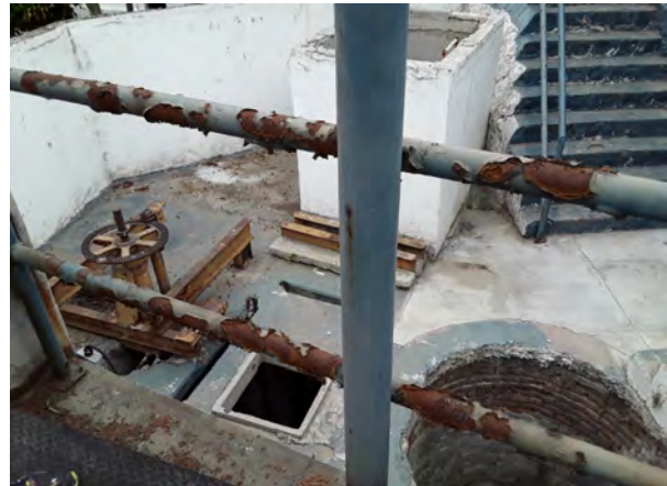
Photograph 4: Corroded conditions of metal handrail at inlet junction box, PB1A&B
