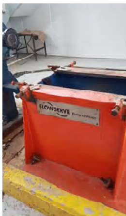
Photograph 11: pump base, while pump out for repair
