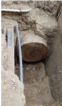
Photograph 7: Steel 36 in outflow from PB CILA to PB-1A
