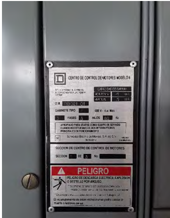
Photograph 37: MCC at PB1A
