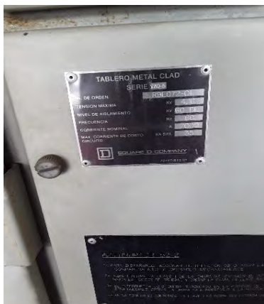
Photograph 35: PB1A MCC plate
