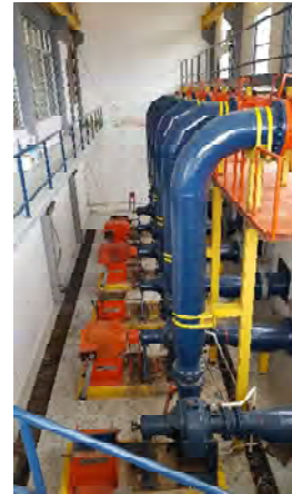
Photograph 8: SAB pump station from open channel to treatment
