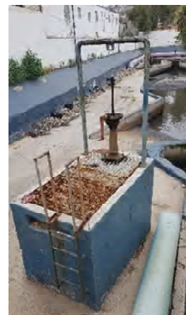
Photograph 18: junction boxes with corroded cover
