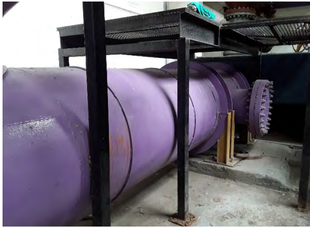
Photograph 21: PB1A effluent manifold
