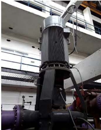
Photograph 19: vertical pump 3B
