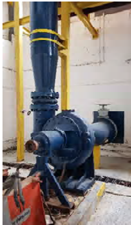
Photograph 15: centrifugal pump setup
