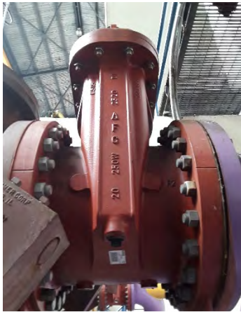
Photograph 9: 20 in check valve stuck
