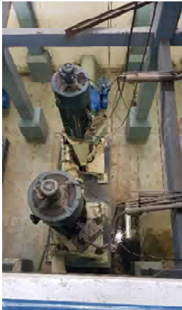
Photograph 37: pump 1 train setup
