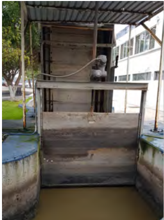
Photograph 7: non-working conditions of screens
