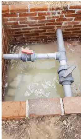
Photograph 21: chlorine injection station
