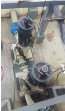
Photograph 38: pump 2 train setup
