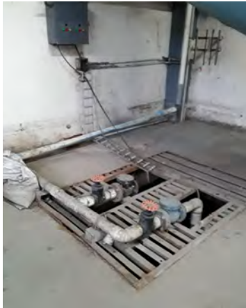
Photograph 31: Sump pump system
