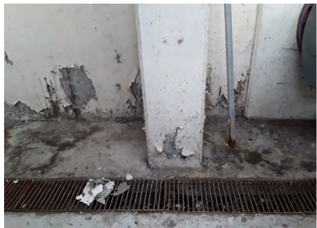
Photograph 24: deteriorated building conditions
