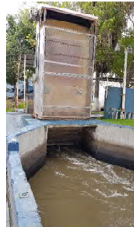
Photograph 16: metal screens with visible corrosion
