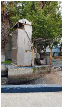
Photograph 15: metal screens with visible corrosion
