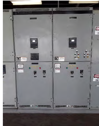
Photograph 38: MCC at PB1A
