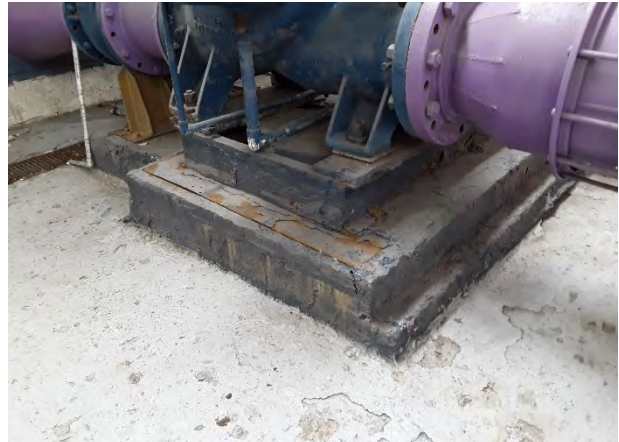
Photograph 32: concrete base deteriorated conditions
