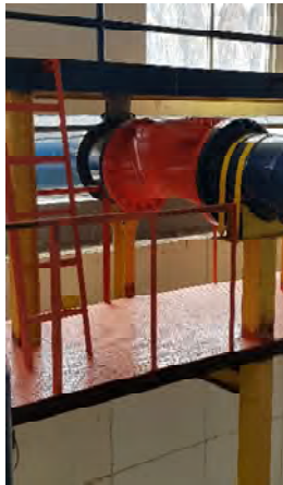
Photograph 9: check valve setup at lift station
