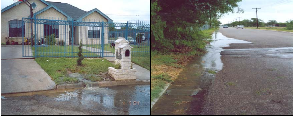
Sanitary sewer overflows in residential areas and streets of the City
